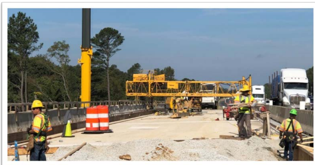
Preparation of the EB Burma Road Bridge for Latex Modified Concrete Overlay
