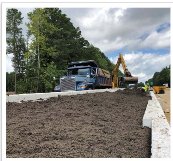
Median barrier backfill in preparation for final Phase II traffic shifts on east end of project
