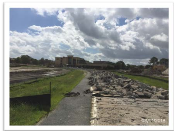
Rublized Pavement Exit 15B Loop
