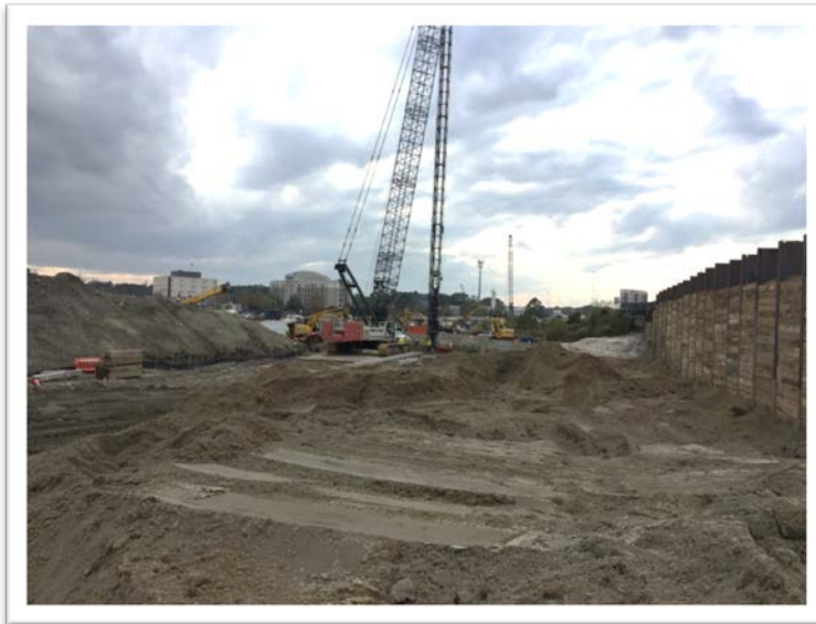
Pile Driving Bridge B-601 with Support of Excavation Wall (right, looking west)
